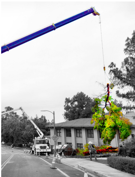
A crane lifts a fallen pine tree. (UCR/Mark Jones)
