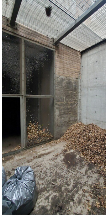
Greenhouse 1 mechanical room. (UCR/Bill Hensche)
