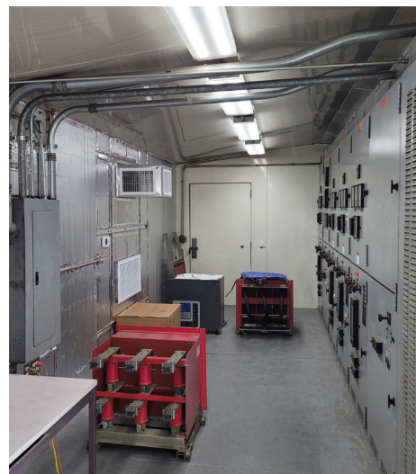
A substation HVAC project reduced peak temperatures of 130 degrees in the summer to now only upper 80s. (UCR/Bill Hensche)
